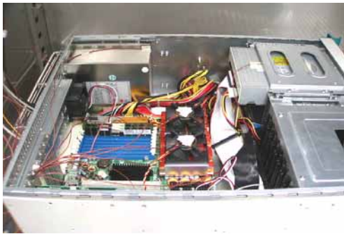
The view of the thermocouples connections.
